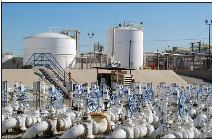
Products Pipelines Watson facility in southern California
