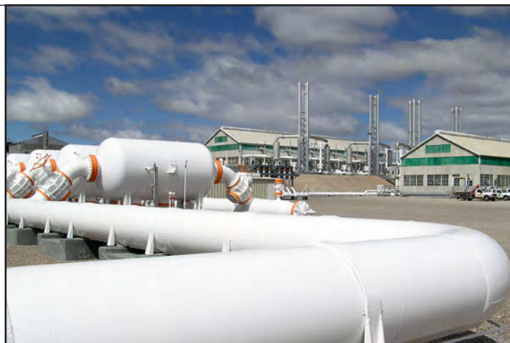
EPNG compressor station in Arizona
